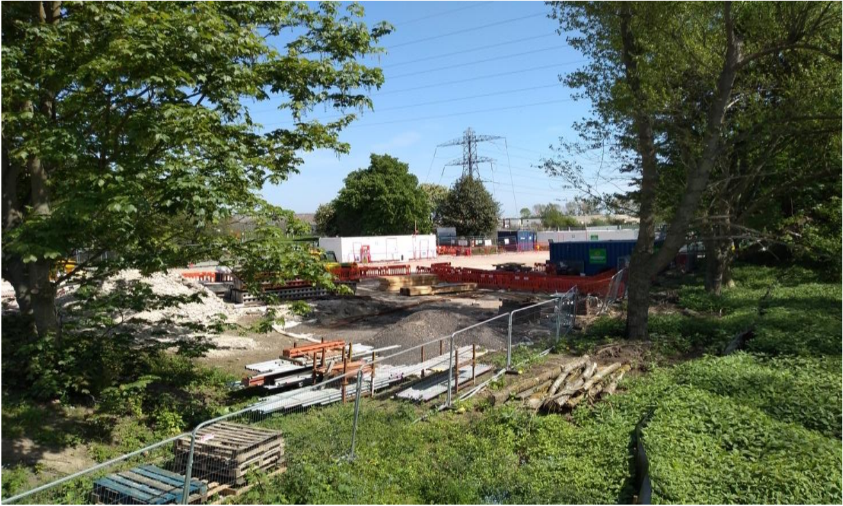
Building work underway North bank Skelton Grange road bridge. Credit: Leeds Cycling Campaign.
